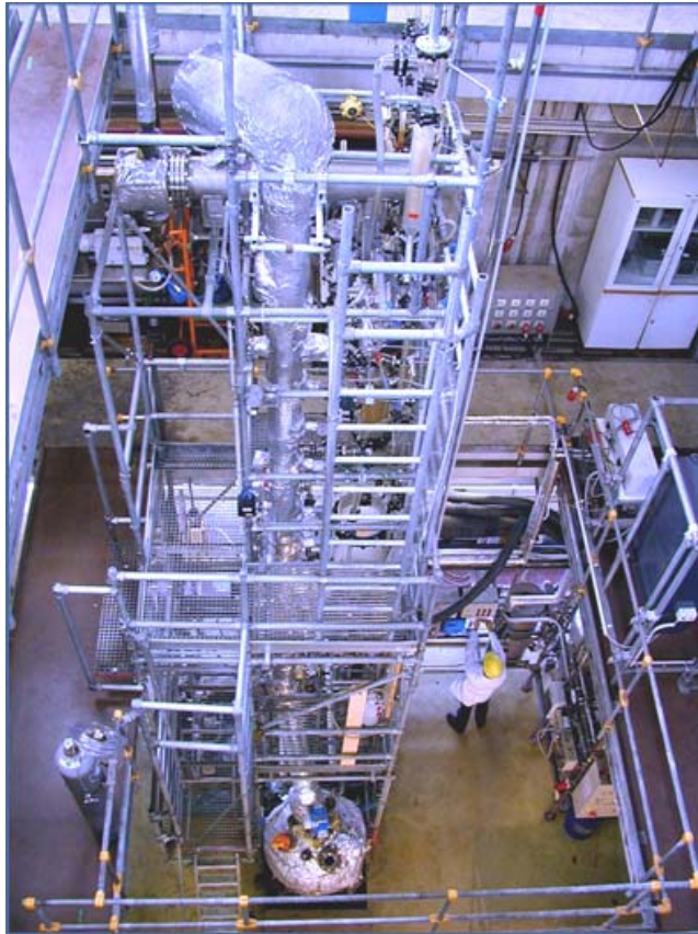
Reactive distillation column
